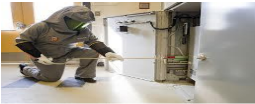
Fig 1: Manually operated to rack in and out
