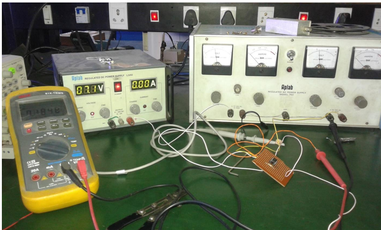
Figure 5 Testing of feedback operational amplifier hardware at Laboratory
