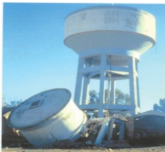
Fig. 1 Failure of the reinforced concrete supporting tower of an elevated reinforced concrete water tank during the 1980 El-Asnam Earthquake, Algeria.
