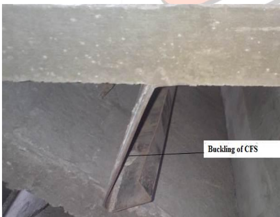
Figure (11): Typical large-scale test specimen (b1) failed due to buckling of CFS at support.
