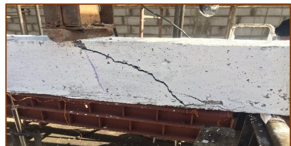
Figure 7 Failure Pattern of Beam
