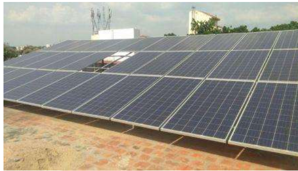
Fig. 2 Solar Modules Array Structure
