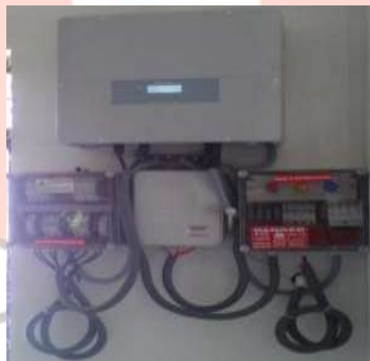
Fig. 3 Assembly of ACDB, DCDB & Inverter
