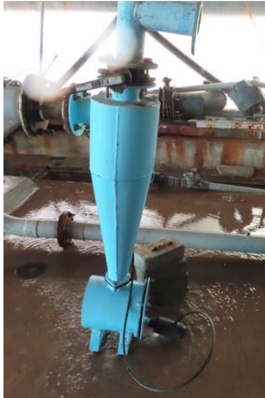
Fig. 08 Drain Valve Set up
