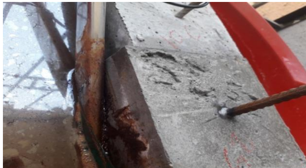
Fig. 2: Deposition of rust on stainless steel bars
