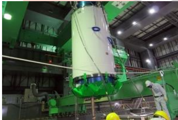
Fig.4. Photo taken by Tokyo Electric Power shows the work progress at the damaged No. 4 reactor building at the Fukushima Daiichi nuclear-power plant
