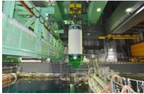
Fig.3. Advanced Automation Technology Using PLC Helped for Removal of Spent Fuel Rods from Unit 4. Source: Tepco/Japan
