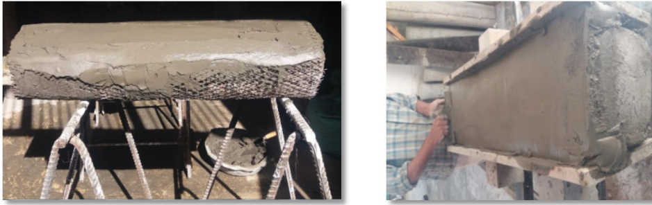
(b) The gap of 10 mm at the top and the bottom of the specimen Fig 8. Columns Confined with mortar Layer
